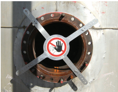
Figure 8: Example barring of confined space entry (reproduced with permission of CableSafe)
